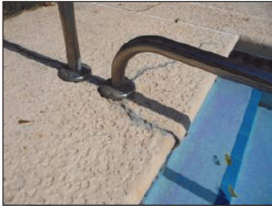
11.2 Picture 5 Cracks in surface area.
