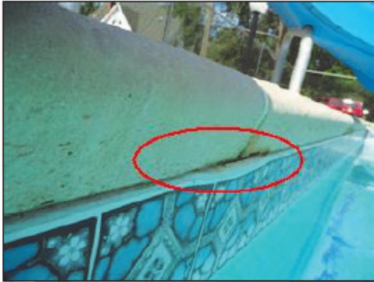
11.1 Picture 1 Liner has pulled loose.
