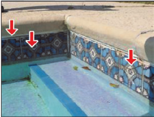
11.2 Picture 1 Pool sides are cracked.
