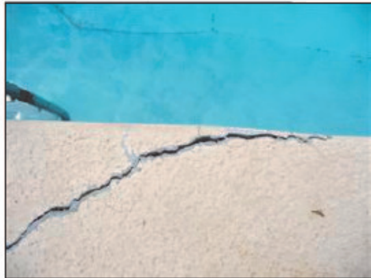
11.2 Picture 4 Deep crack in pool perimeter.
