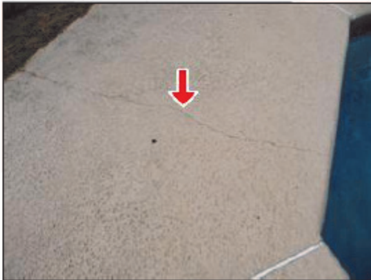
11.2 Picture 3 Crack in surface.
