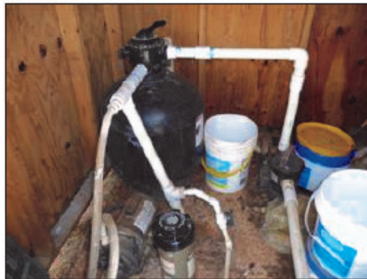
11.0 Picture 1 Filter and pump.
