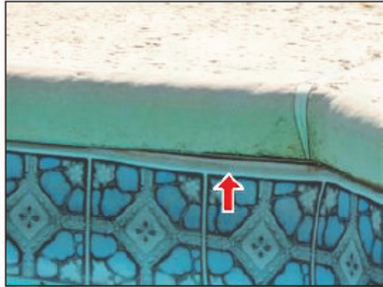
11.1 Picture 2 Liner defect.
